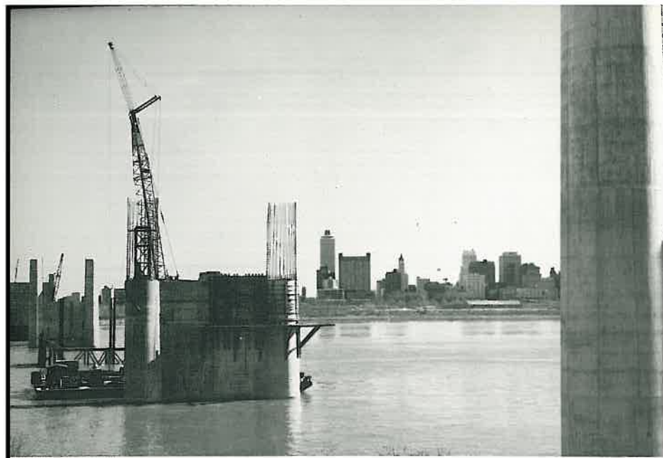
A portion of the Memphis skyline is seen through two of the eight main channel piers.
