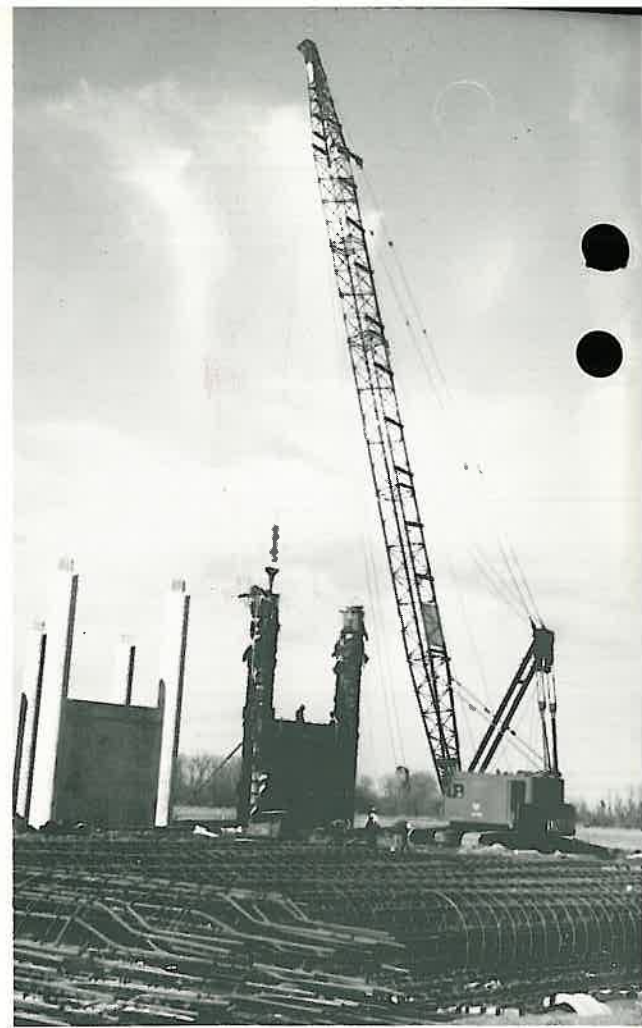
Main column reinforcing steel is woven into spiral cages before being dropped into the pier forms. After the steel is set in place, concrete is poured around it to form the columns on each end of the pier.
